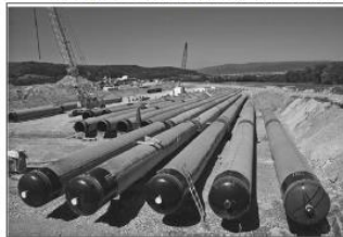
NG Pipe Storage, Erdgas, Switzerland
